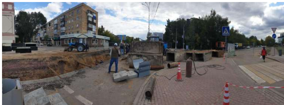
Fig. 5 – Situation at the intersection of Komissarova Street and Voinov-Internatsionalistov Street during the overhaul of utilities
